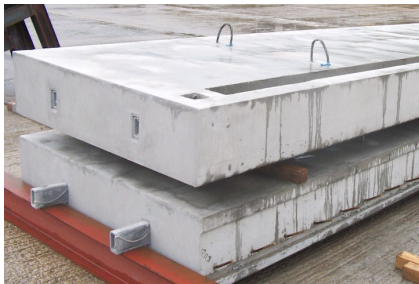
DTS in floor units
