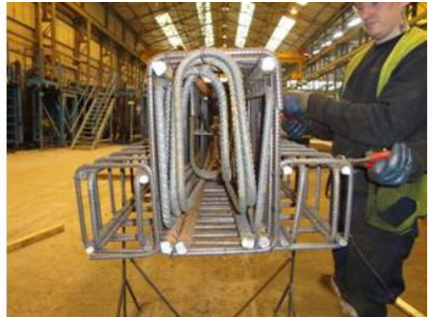
4.2 Ready for insert the beam unit, note the strips in top of the saddle bars, makes it easier to insert the BSF
