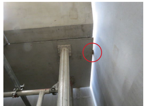
RVK connectors (e.g. circled) support precast landings off core walls prior to grouting
