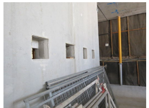
Outside of the stair core showing recesses built into the twin wall
