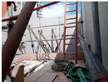
Pockets in twin walls ready to receive RVK connectors at The Whiteley
